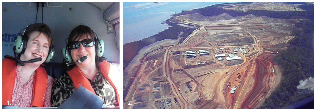
1. Senior Representative Karen Hooper (left) and Economist Marileze van Zyl of the Queensland State Office, on board a helicopter over Curtis Island 2. A view from the helicopter of one of the LNG plants under construction on Curtis Island
